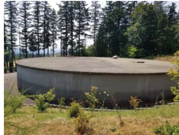
This is the District's 3.0 MG reservoir. It is built to current earthquake design standards.
