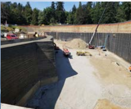
This is Portland's project to replace the uncovered reservoirs at Washington Park. West Slope will pay a portion of the construction costs through our water rates beginning in 2023.
