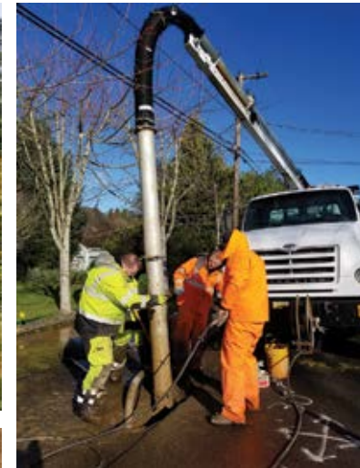
Field crew excavating with a VAC truck to expose a leak in the District's water main. If customers see this truck out on the street, chances are we are repairing a water main break as quickly as possible. Please drive safely around our field crew.
