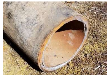
Water pipe cut showing condition of pipe.
