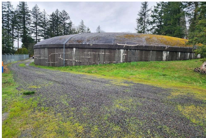
Picture of the District’s Reservoir #2 (2.25 MG of storage), built in 1961 and not earthquake resilient.
