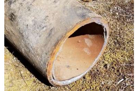
Water pipe cut showing condition of pipe.
