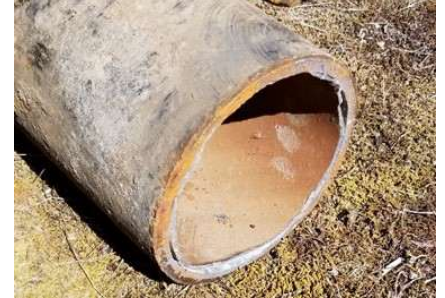
Water pipe cut showing condition of pipe.
