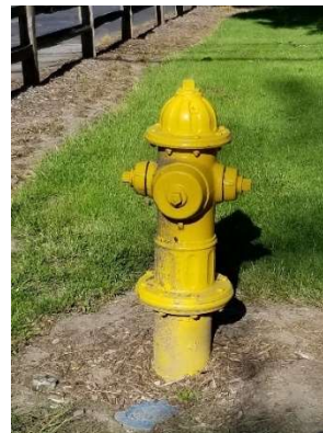
District fire hydrant.
