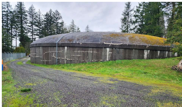
Picture of the District’s Reservoir #2 (2.25 MG of storage), built in 1961 and not earthquake resilient.
