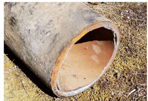
Water pipe cut showing condition of pipe.
