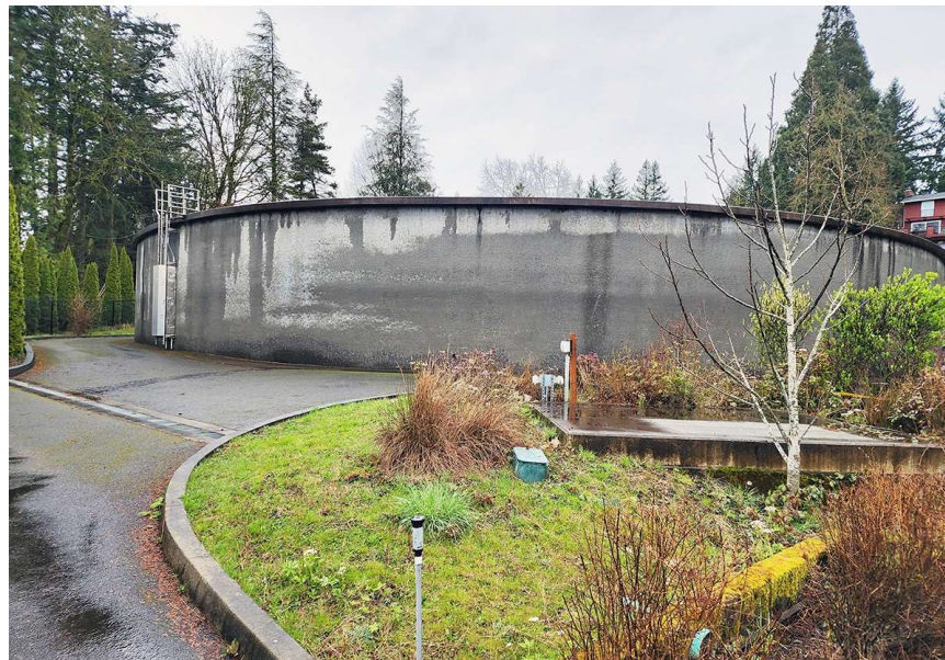
Picture of the District’s Reservoir #3, when it was completed in 2009.
